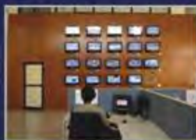
Command and Control Centre
